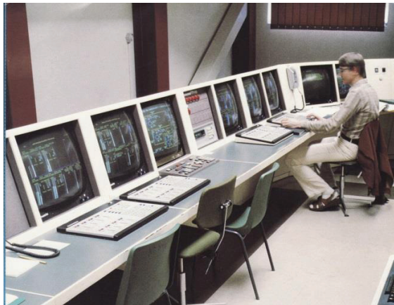
A Damatic control room
